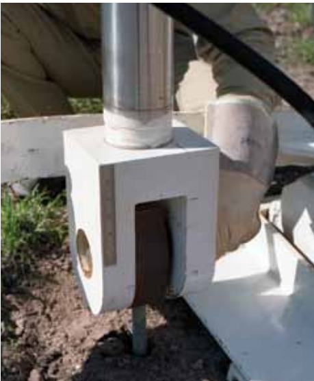
Hydraulic pull test unit.
